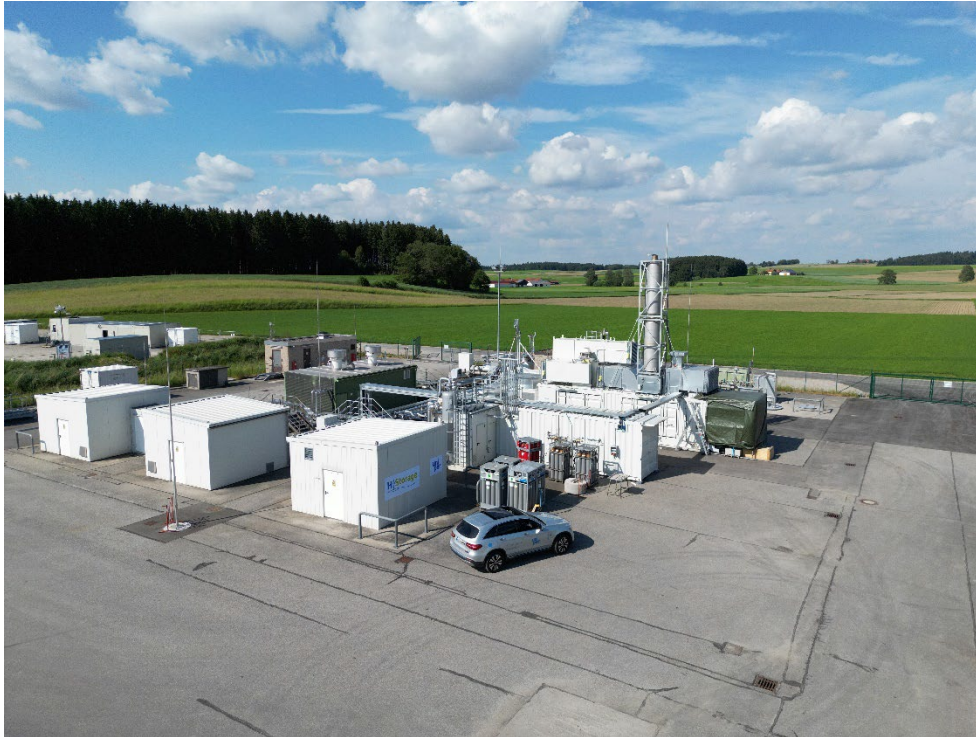
The HyStorage research project is being carried out at the BW B6 drilling site at the Bierwang storage facility. (Source: Uniper Energy Storage)
