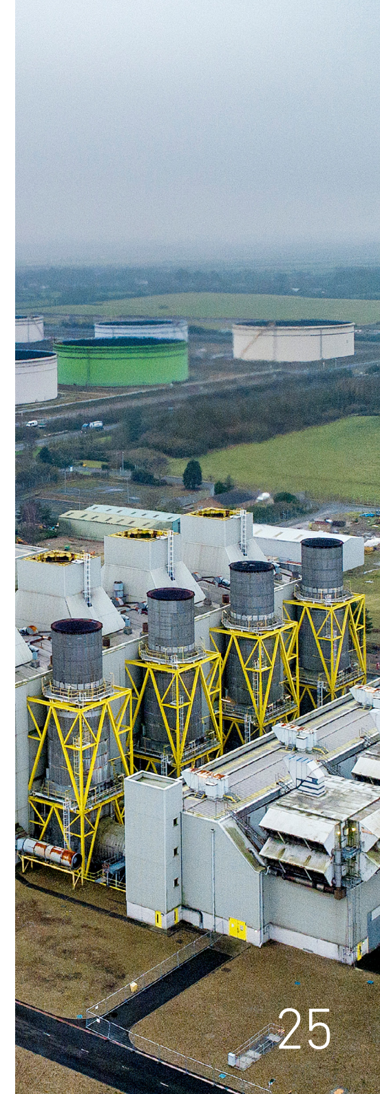
Killingholme power plant
