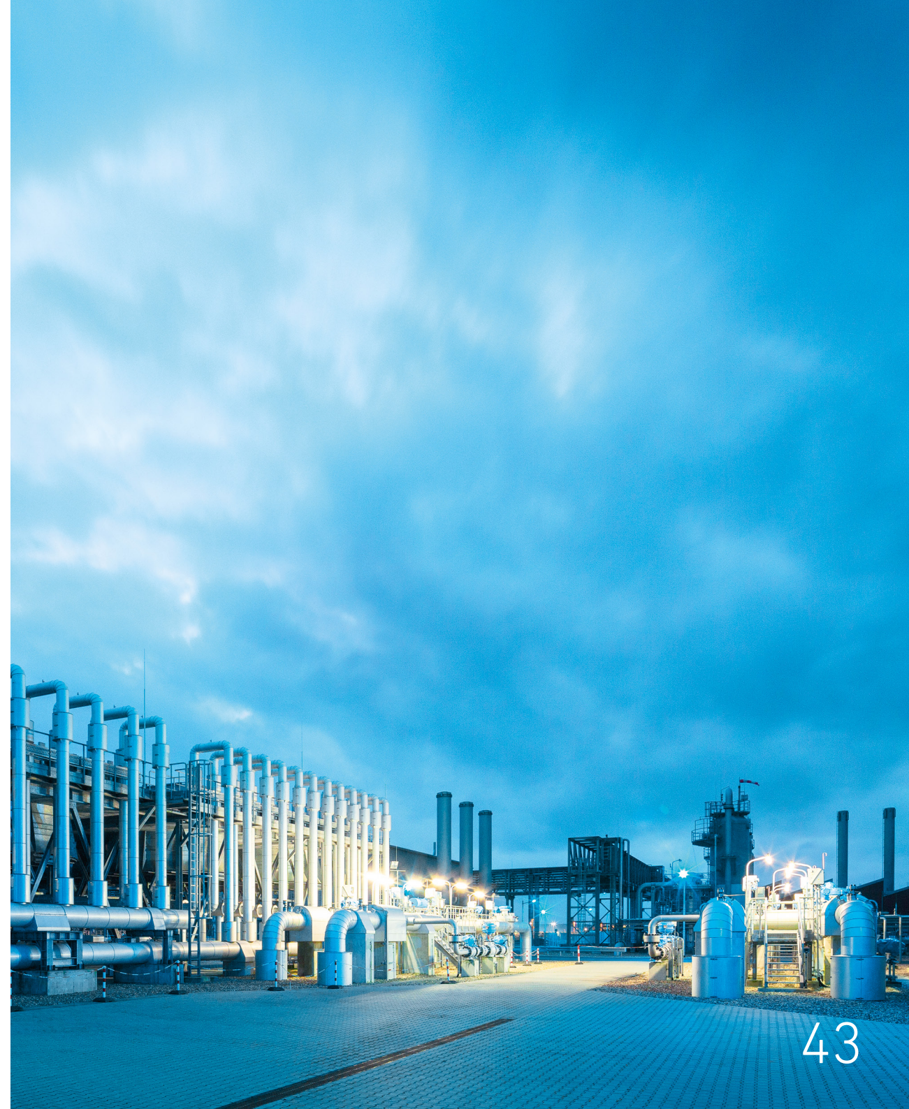
Etzel natural gas storage facility
