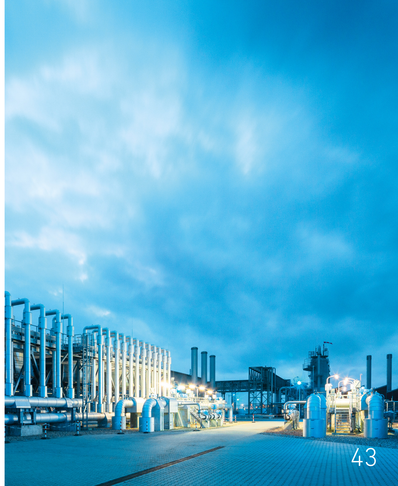
Etzel natural gas storage facility
